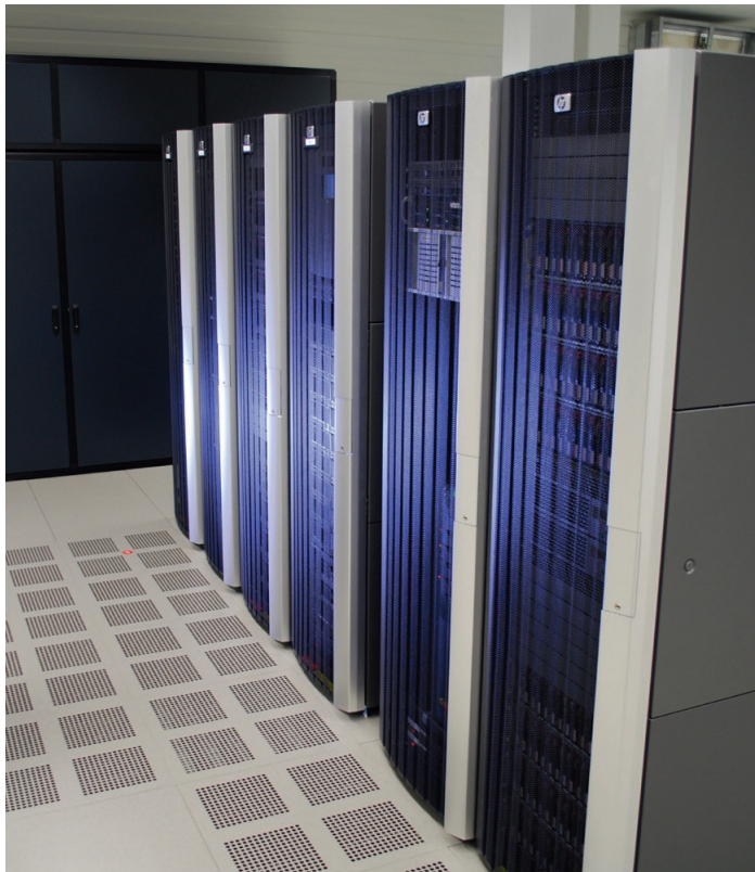
The data center servers require the highest level of security.
