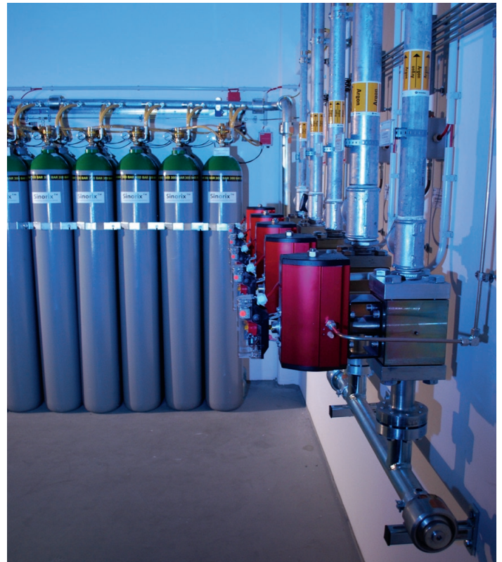
Sinorix extinguishing solutions with natural agents can be customized to optimally meet data center requirements.
