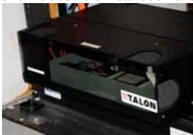
A TALON Network Manager mounted in one of Noridian's IS closets.
