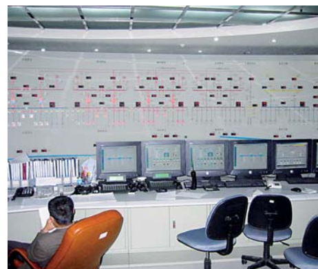
Command control center
